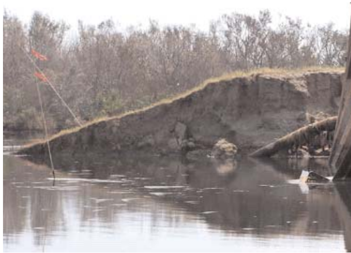
Levee Break Photo: Louisiana Department of Environmental Quality
